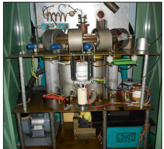
Fig. 2. The external view of the high voltage generator after the upgrade
